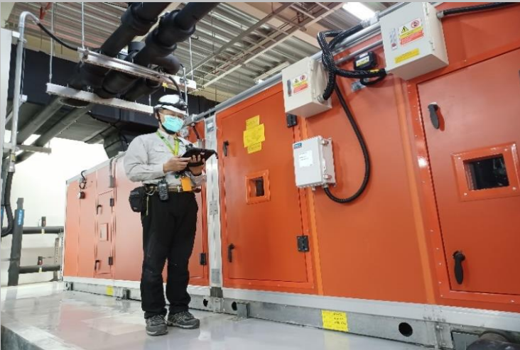
Air handling unit maintenance
